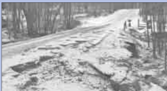
Hayden Hill Road washout about 100 yards from the North Road intersection.
