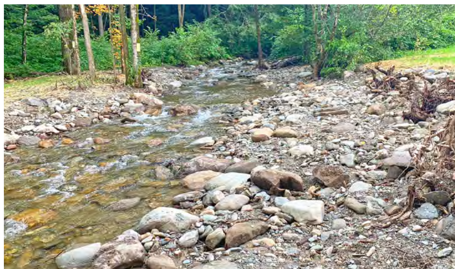
Area above Sugarhouse Lane, after construction, where old bridge abutments were removed, and the floodplain was restored. Photo credit: Alex Marcucci, SLR
